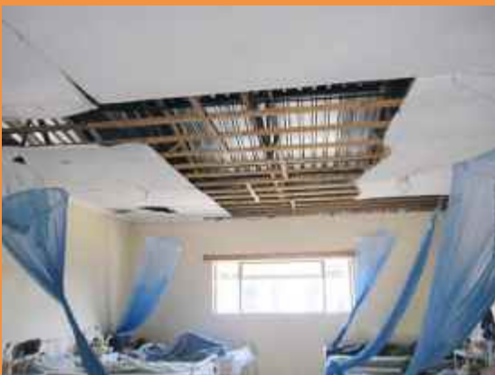
A dilapidated (and dangerous) hospital ward
