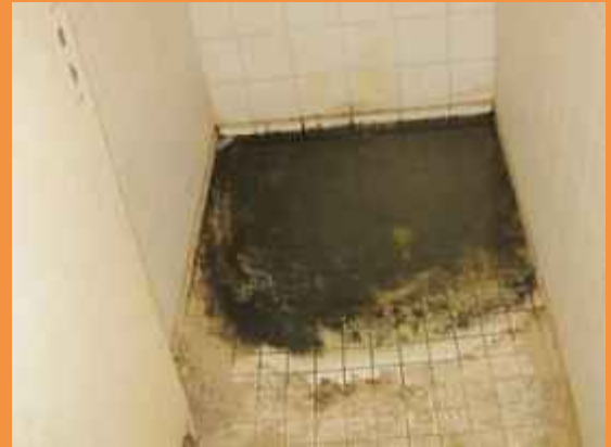
A broken and blocked shower
